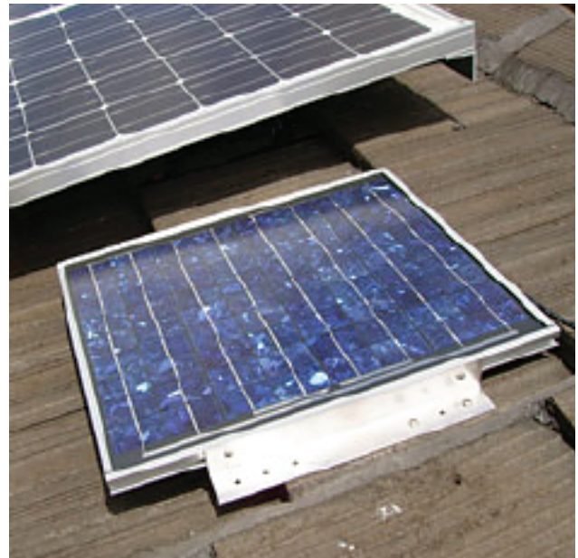
remote solar panel installed on roof
